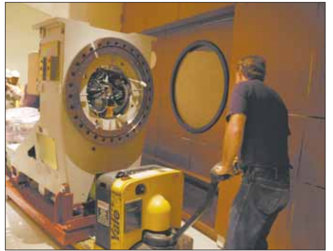
One of three new linear accelerator radiation treatment machines is moved into place. Each unit weighs almost 40-thousand lbs.
