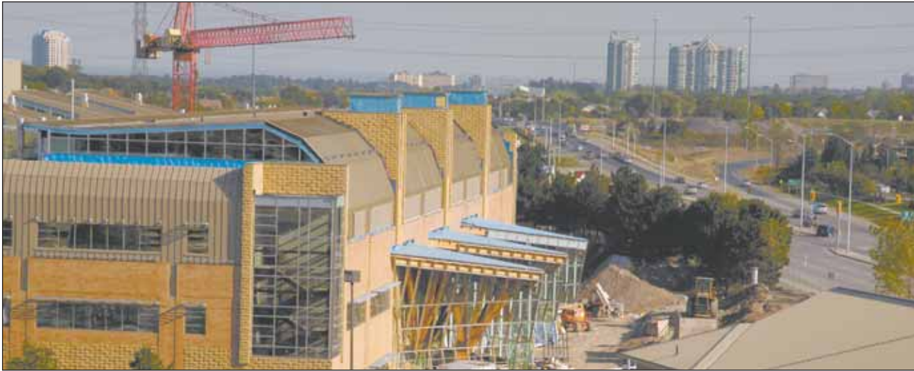
Construction continues to progress at The Credit Valley Hospital where The Carlo Fidani Peel Regional Cancer Centre and Ambulatory Care Centre are scheduled to open this spring.
